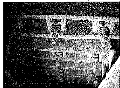
Figure 10 Dust agglomeration underneath the grate of the clinker cooler
