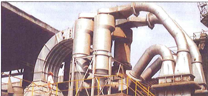
Figure 3: the HURRICLON installation at Colclinker
