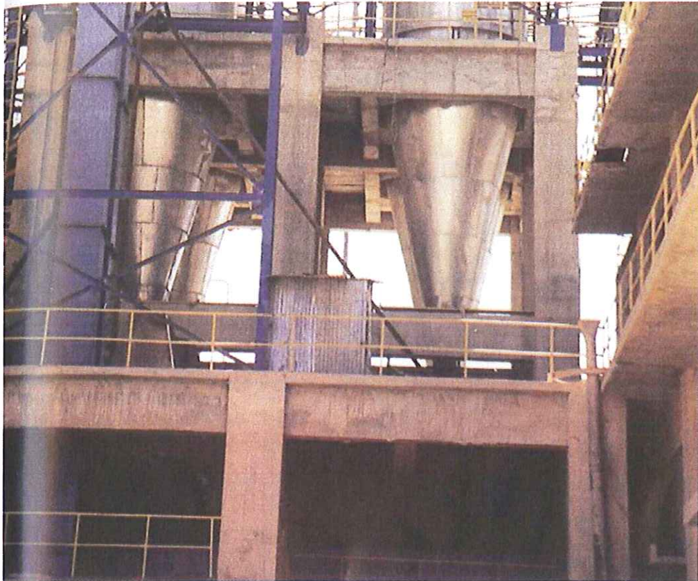
Fig 5. Raw mill cyclones after HURRICLON
