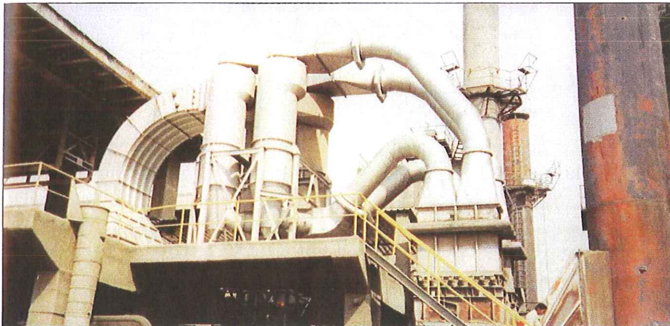
The HURRICLON® installed in the Colclinker plant.
